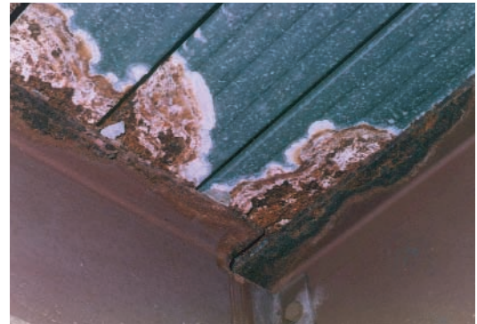
Figure 1: Corroded concrete decking showing the result of sub-standard expansion joint and finish detail.
