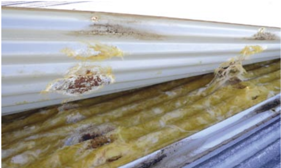
Figure 3: Photo depicting moisture penetration due to the absence of a vapour barrier in a tropical environment.
