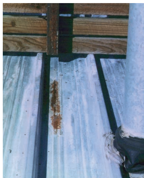
Figure 1: CCA Treated Timber Walkway
