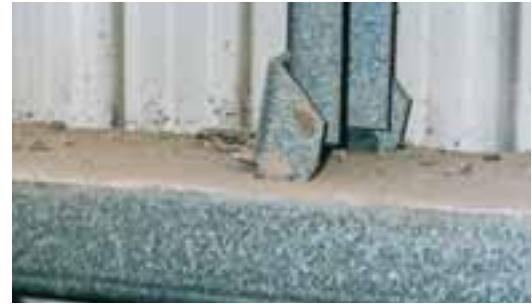
Figure 2: Build-up on purlin
