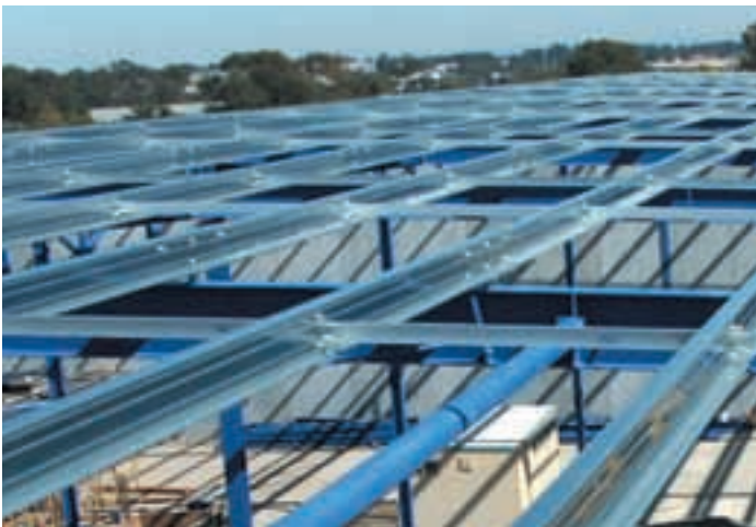
Galvanised steel purlins
