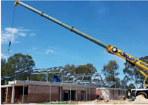
ABOVE: A construction scene at the centre, where the exposed skeleton of the roof shows the complexity in the design. CHS, RHS, SHS and EA in various widths were used to construct the shape, with no two pieces the same. (Image supplied by A Class Engineering.)
